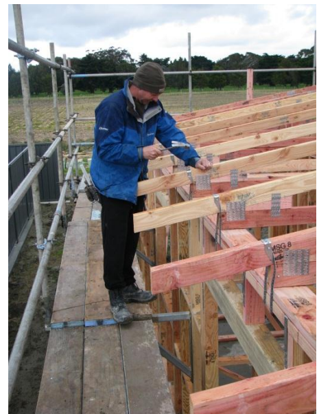
Figure 8: Scaffolding and brackets can be effective roof edge protection.
