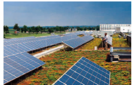
6. Roof with fully-installed solar energy system.
