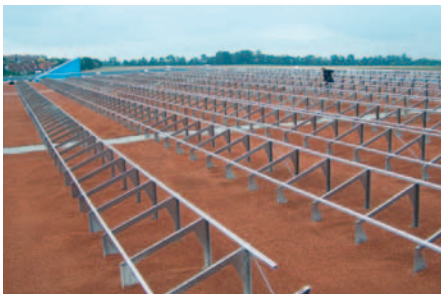
4. The Solar Bases are covered with system substrate as per the required load.
