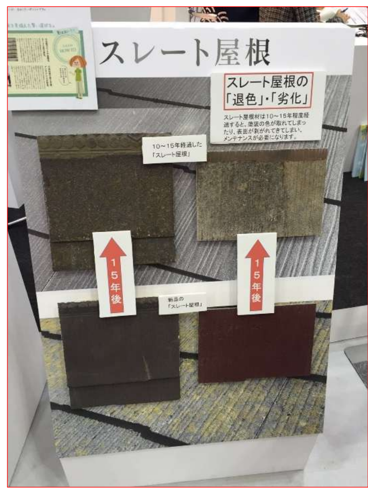
Others Roofing materials after 15 years
