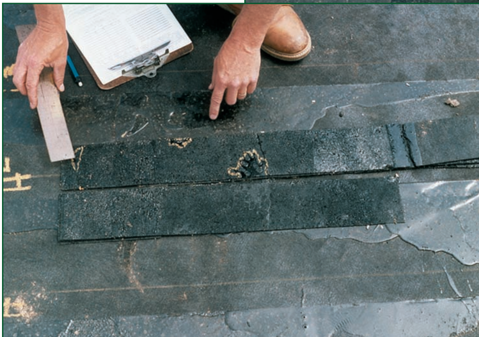
Photo 10: Interply voids or lack of continuity in mopping.
