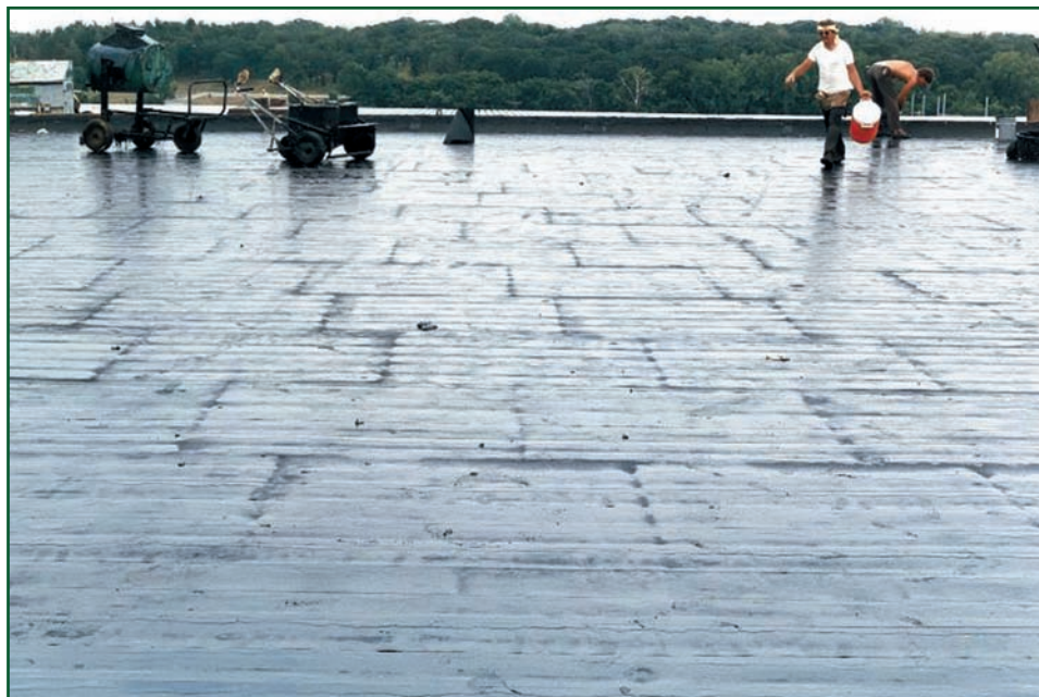
Photo 6: Results that can be anticipated when application temperatures are well above the product's EVT. Note the "picture framing" as a result of excessive temperatures and bleed-through at joints in the insulation.
