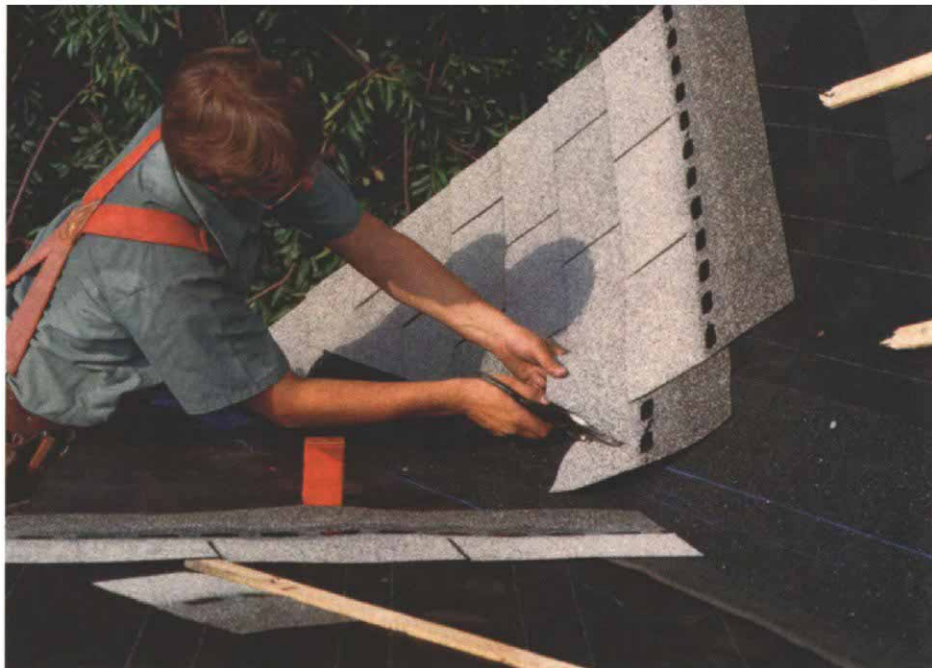
Working his way up an open valley lined with mineral-surface roofing, Smith uses tin snips to trim shingles flush with the chalkline. Blue chalk is preferred because it washes away in the rain; red chalk will permanently stain the shingles.
